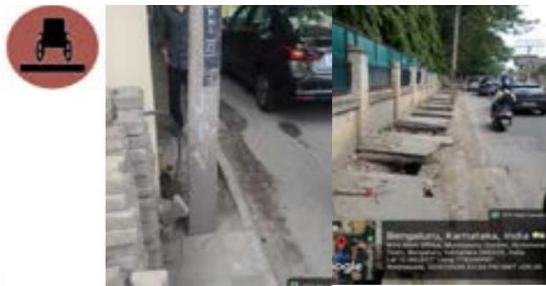
3.1 Footpath Infrastructure, Kerb and Level Differences: Narrow and uneven pedestrian walkway with a utility pole obstructing the usable footpath width. Footpath is severely damaged with open drainage and broken pavement, creating significant level differences and reducing pedestrian accessibility.
