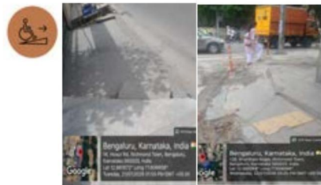
3.2 Ramps and Transitions: Ramp/transition is provided at the road edge, but the surface is uneven and does not provide a smooth accessible connection. Tactile paving is present near the transition; however, the surrounding surface is damaged and the accessible route is interrupted.
