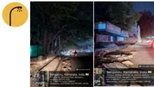
3.9 Lighting Conditions: Pedestrian edge and footpath are poorly illuminated at night, with heavy tree cover further reducing visibility. Night-time visibility is inadequate along the damaged footpath, creating potential safety concerns for pedestrians.
