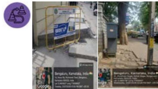
3.10 Barriers, Obstructions and Encroachments: Temporary barricades obstruct the footpath and force pedestrians to negotiate around the obstruction. Tree roots, broken paving and utility infrastructure obstruct the pedestrian pathway and significantly reduce its accessibility.
